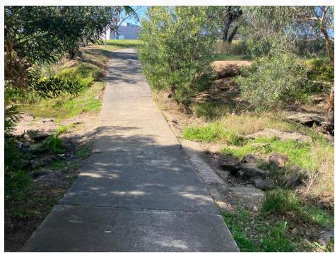
Path crossing over Toolern Creek in poor condition.
